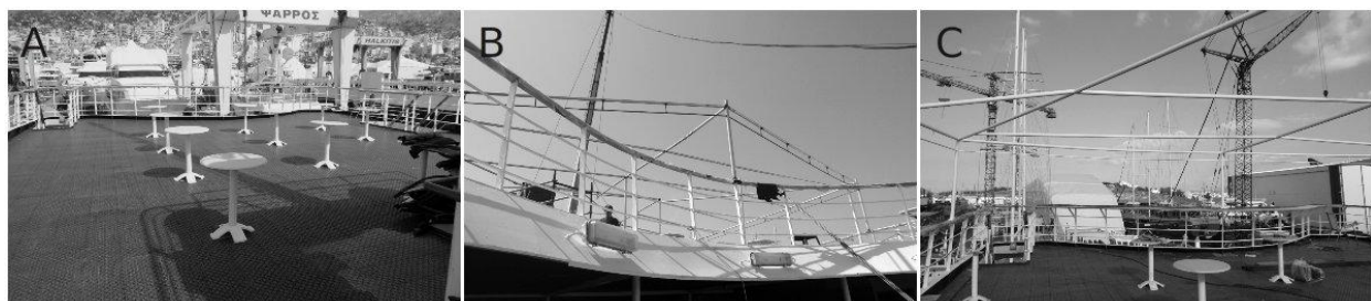
Figure 9a, b, c. Upper Deck Back Side Rail, Existing Situation. Source: Siniša Prvanov.
