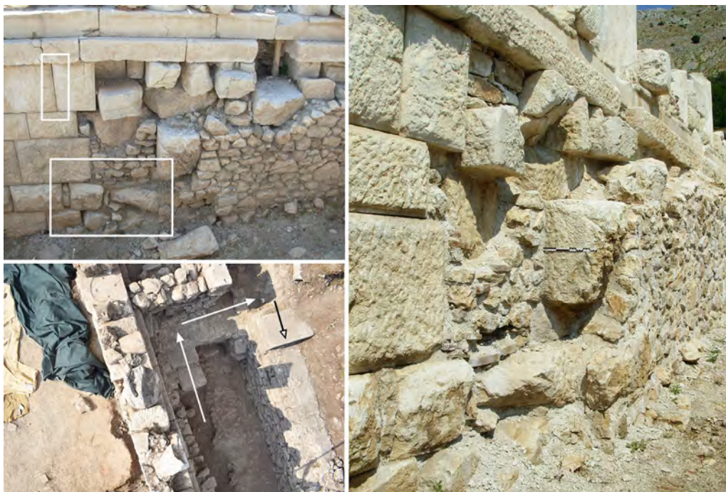
Fig. 42. (upper left) Eastern view of the location where a makeshift extension was placed against the Hellenistic wall. Indicated are the widening of the joints and eastwards protruding blocks indicative of the collapse of the original continuation or extension of the wall. (right) Southeastern view of the same situation, clearly displaying the mortared rubble support wall. (lower left) Top down view of the northern extremity of the extension, including the stairway.
